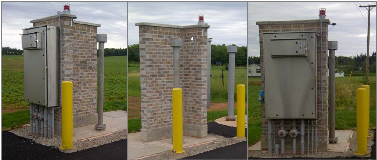
Figure 5-9 Example of a Weather Proof Enclosure for Exterior SLS Electrical Components
