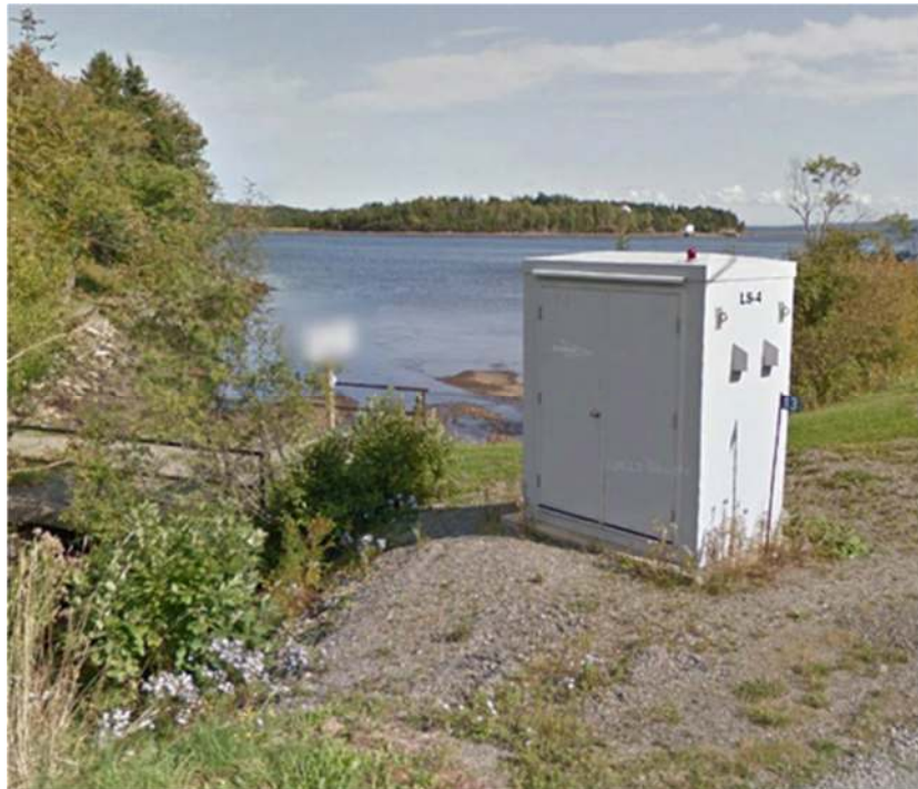
Figure 5-13: (4) Church Street Extension Sewage Lift Station – Guysborough
